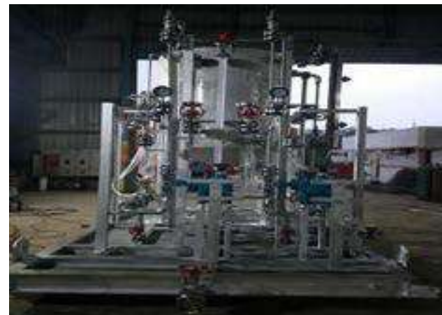
Chemical Injection Skid
