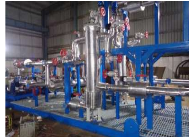
Hot Oil Skid
